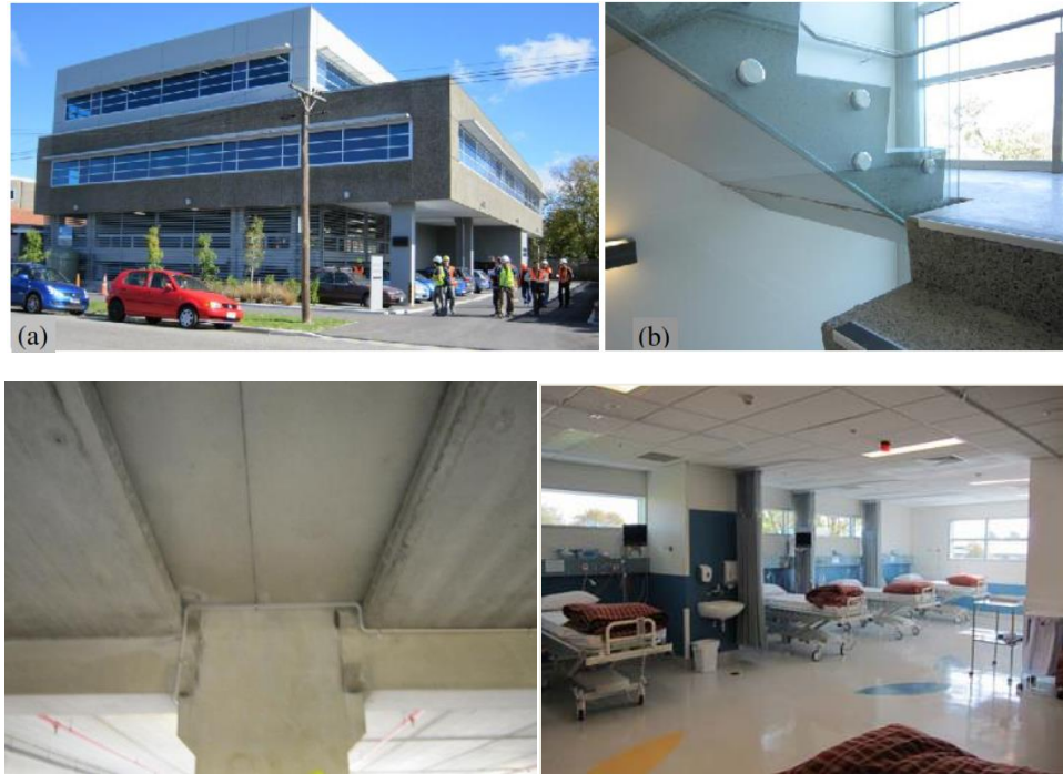
Figure 14: Precast Hybrid Structure [62]: (a) Exterior; (b) Seismic Damage; (c) Frame; (d) Post-EQ Operational.
