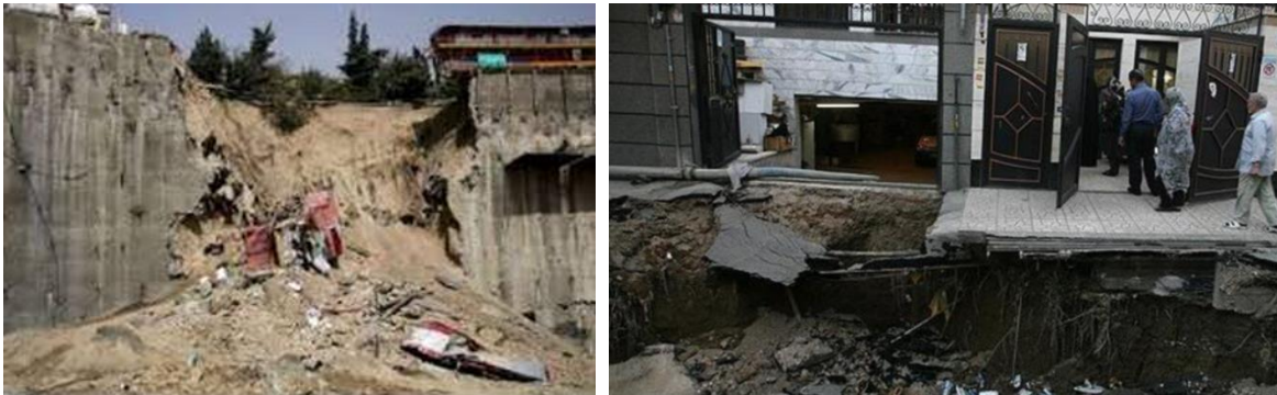
Figure 12: Examples of collapse of such excavations, from lecture by Prof. Fakher of Teheran University [6].
