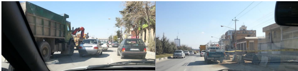
Figure 2: Utility construction on two sides of a Shiraz Boulevards at the same time.
