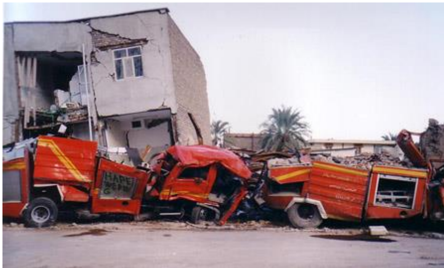
Figure 2: A fire station heavily damaged by the Bam earthquake [5].
